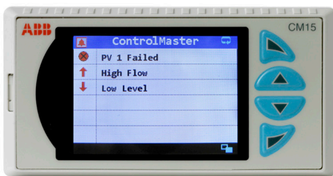
Figure 4 Alarm status display
